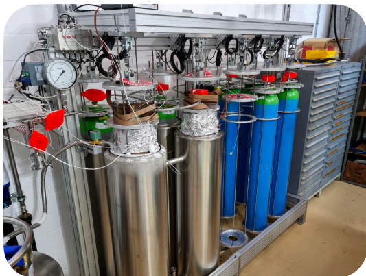
Assembly Storage Array
