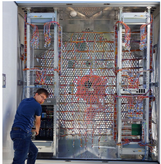
FIG. 6.3 – Camera rear doors open. The safety and power cabinet at the left lower rack position is being inspected. The slow control drawer is installed in the middle of the right rack. Fan drawers and heat exchangers can be noticed at top and bottom of the two racks.
