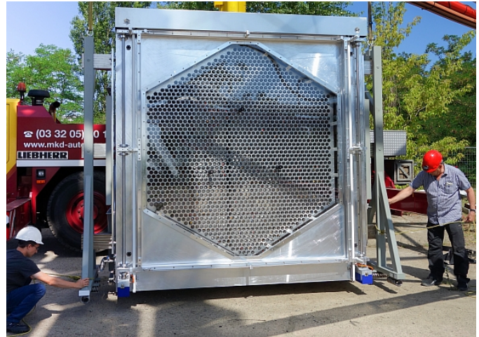
FIG. 6.1 – FlashCam body in Adlershof before installation.
