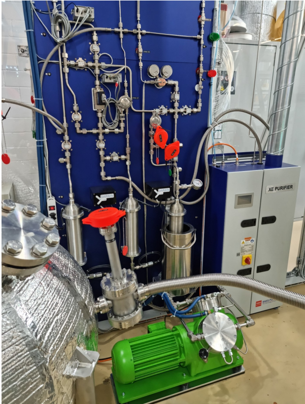
Figure 3.6: Purification gas panel. The gas handling system is seen attached to the back of the panel. The hot metal getter inside its cabinet can be seen on the right. The green pump in front of the panel is the GXe compressor. BoX (section 3.3.4) can be seen on the left.
